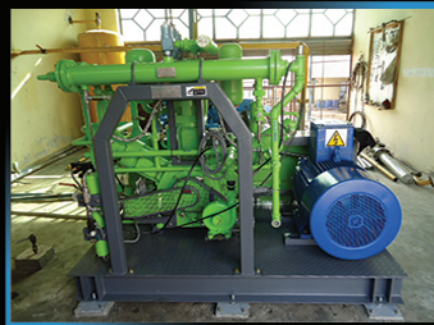
Save CNG Station, Gujjar Khan
